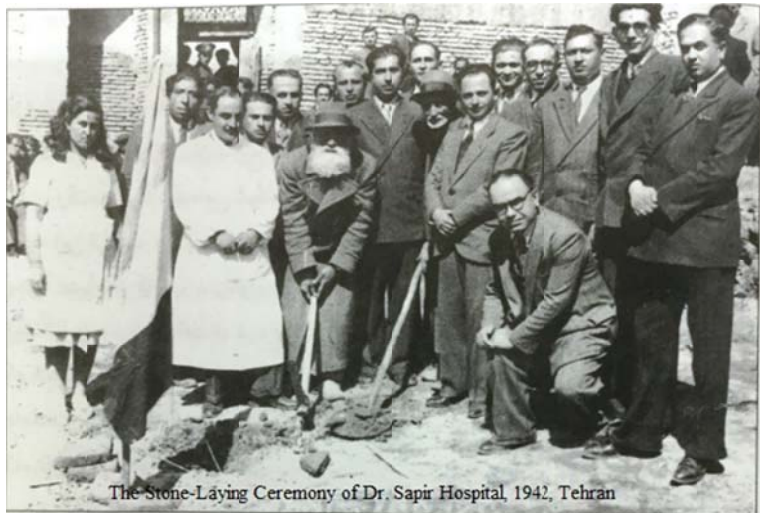
1942, Tehran. Hadji Yeshou'a, middle, holding a pick mattock, leads the stone-laying ceremony of the building.
